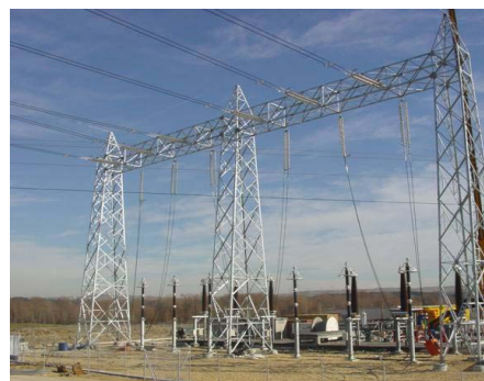
Figure 5: Overhead line cables transition station (400kV)
