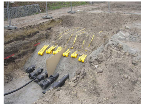
Figure 3: 220 kV cable system pulled in pipes and buried
